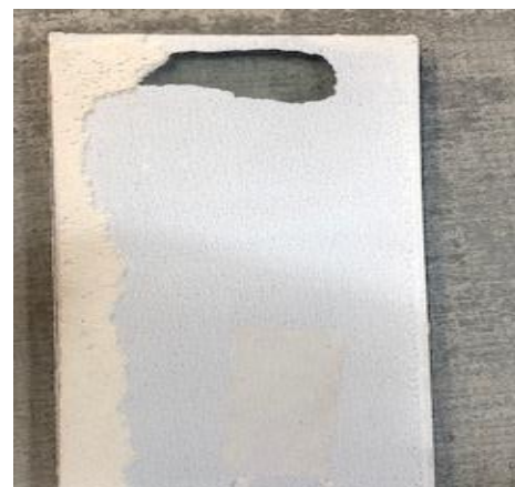
Glass Tile Coating Peeling
